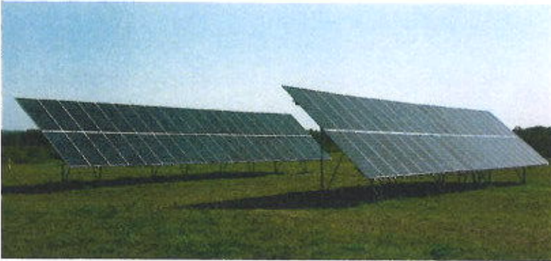
Detroit Lakes Public Utility's 29.3 KW Select Solar Community Solar Garden Detroit Lakes, MN
