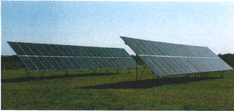
Detroit Lakes Public Utility's 29.3 KW Select Solar Community Solar Garden Detroit Lakes, MN
