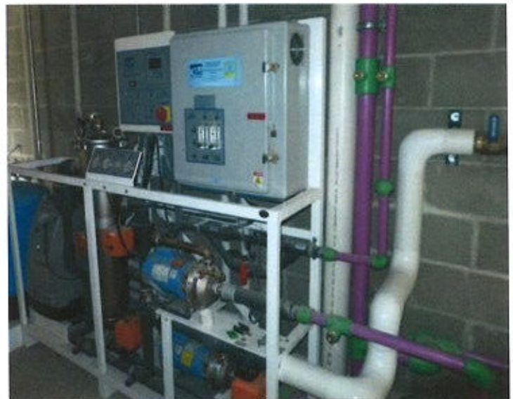
Figure 25. The purple pipes indicate reuse water. A Plumbing Board variance is required for indoor water reuse other than non-potable rainwater catchment systems. This reuse system is located at the new Vermillion State Park sanitation building and is used for toilet flushing.
