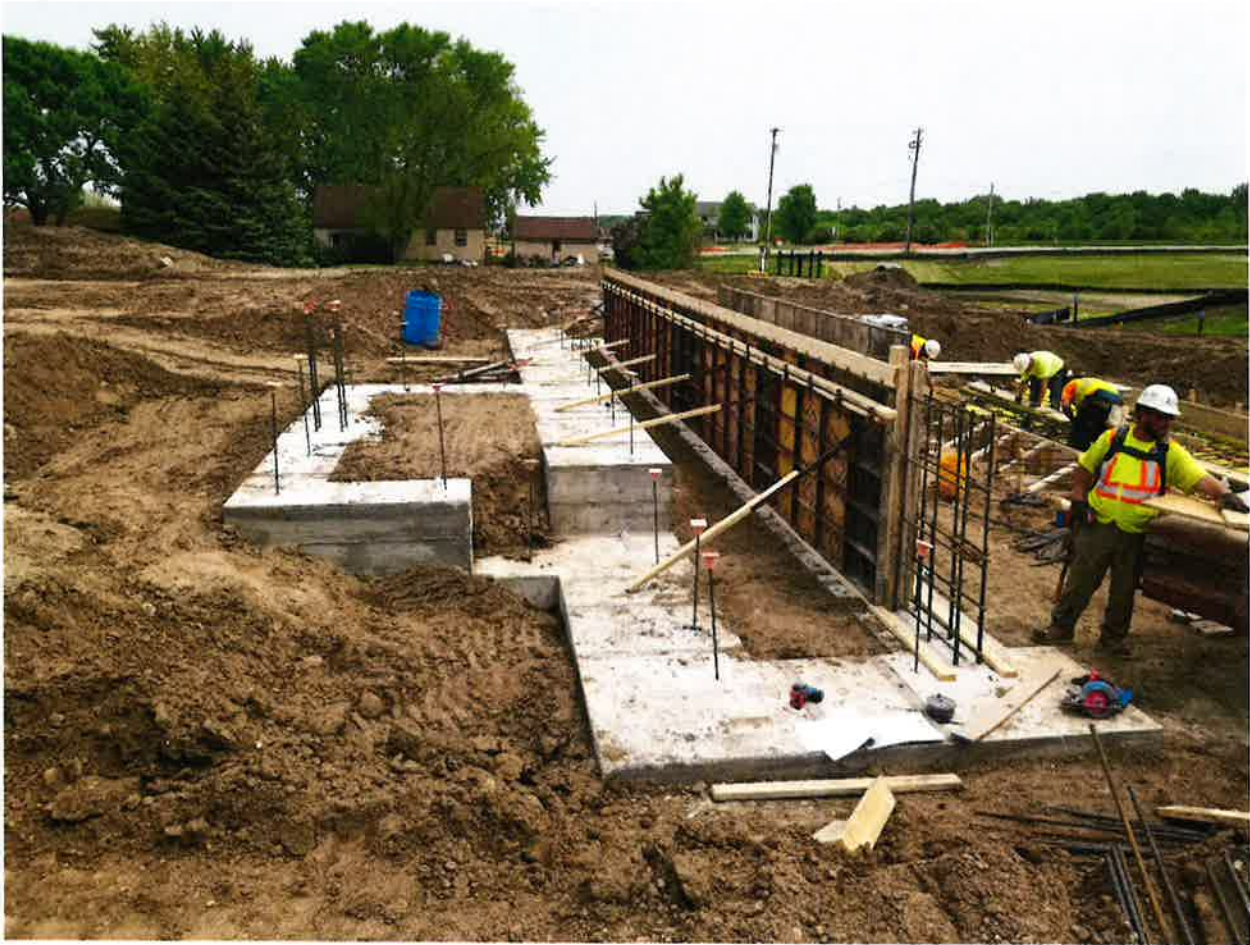
This is the view looking East. What is seen here is the footings that the precast walls are to sit on. The footing extending to the left in this photo is the stoop for the main entrance.
