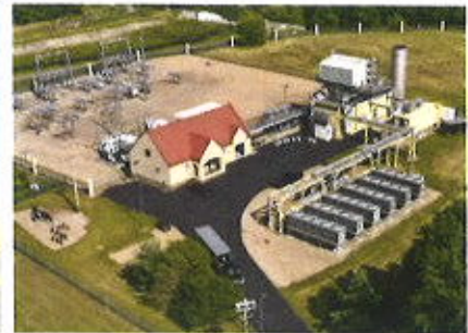
MINNESOTA RIVER STATION CHASKA, MN 49 MW, NATURAL GAS
