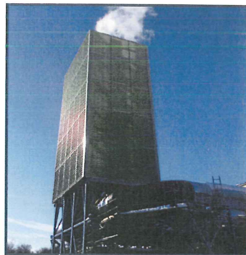
SEP First Fire of Engines - December 9, 2016
