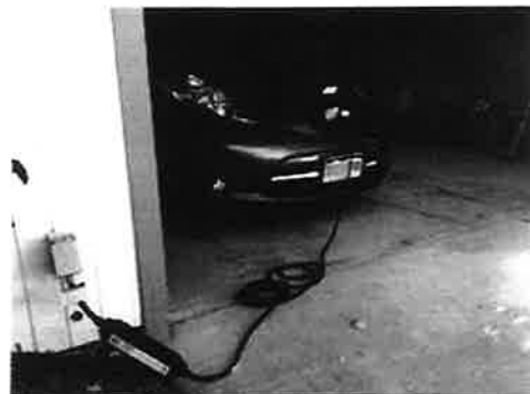
PHEV and EV owners may install Level 2 (electricity_infrastructure.html#level2) (240 V) charging equipment in their homes for a faster charge, or opt for the Level 1 cordset provided with the vehicle as shown here.
