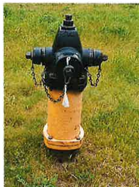
SPU identified Private Hydrant with white "P" and locator ribbon
