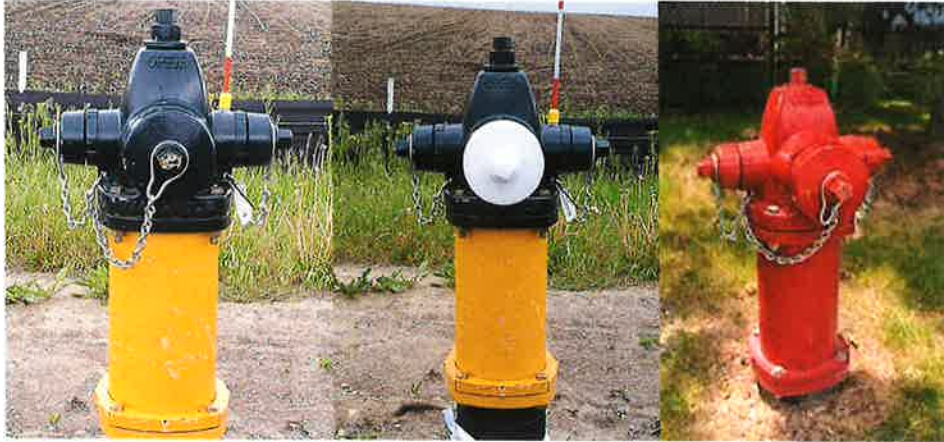
Public Fire Hydrant
