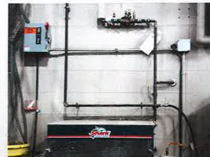
Isolation Backflow Assembly
