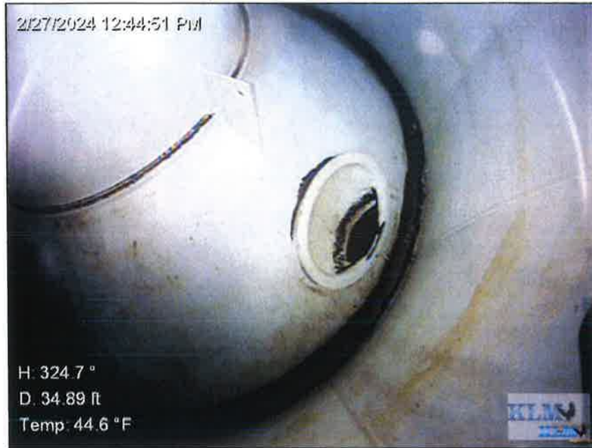
Photo No. 19 Bowl coating conditions Manway visible
