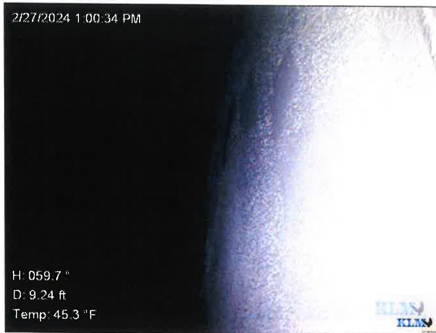
Photo No. 14 Shell coating conditions
