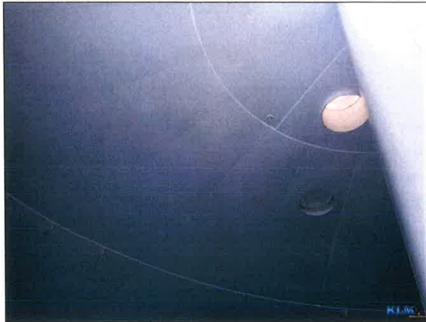
Photo No. 3 View of interior wet roof
