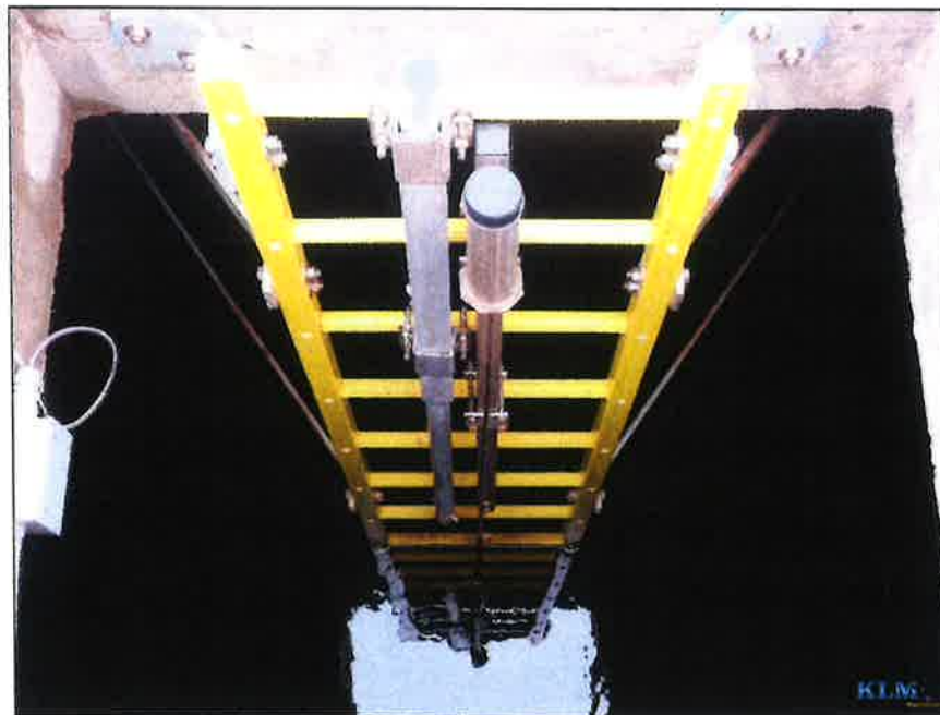
Photo No. 2 Interior wet ladder conditions
