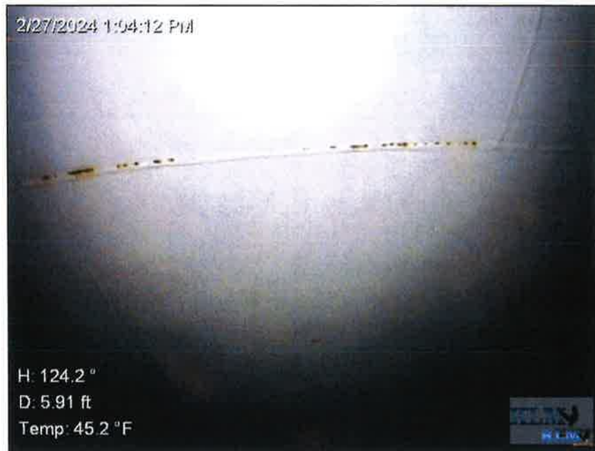
Photo No. 12 Shell coating conditions Pinhole corrosion visible along weld seam
