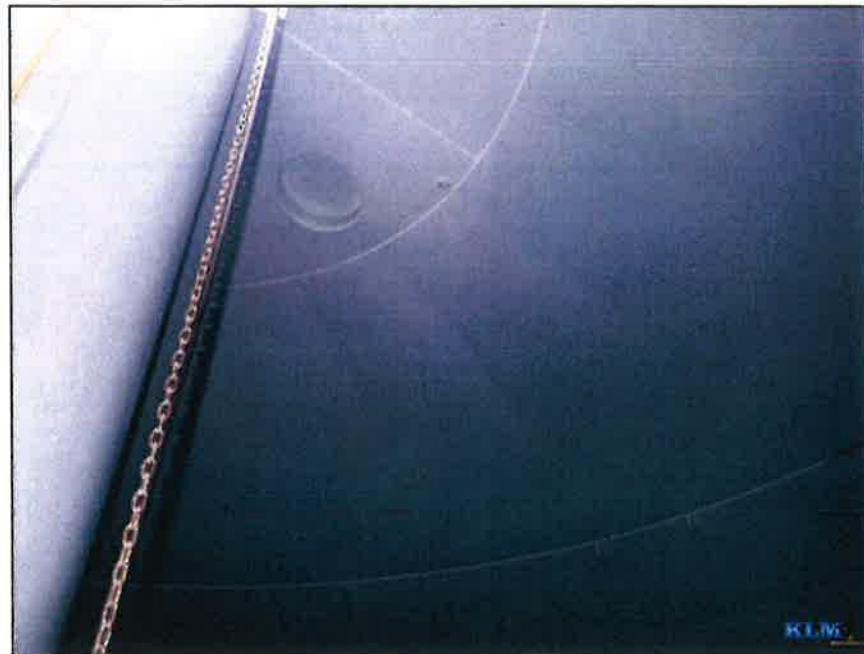
Photo No. 4 View of interior wet roof
