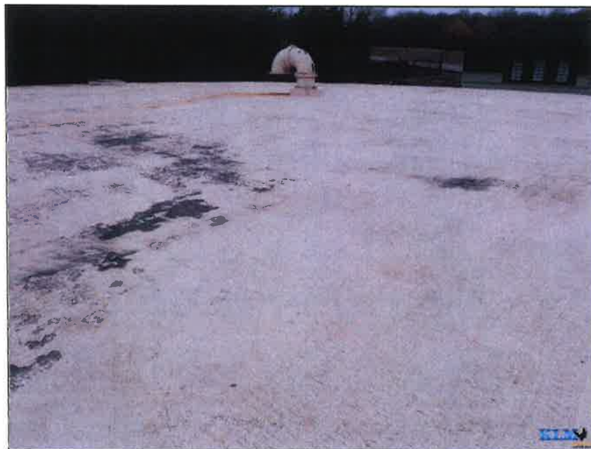
Photo No. 10 Condition of roof coating
