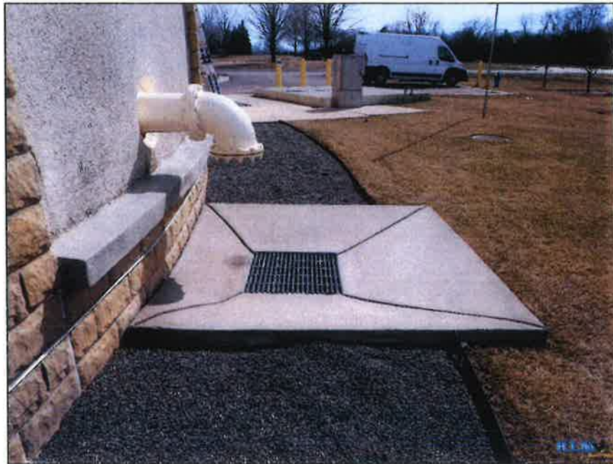
Photo No. 19 Overflow pipe discharge and catch basin
