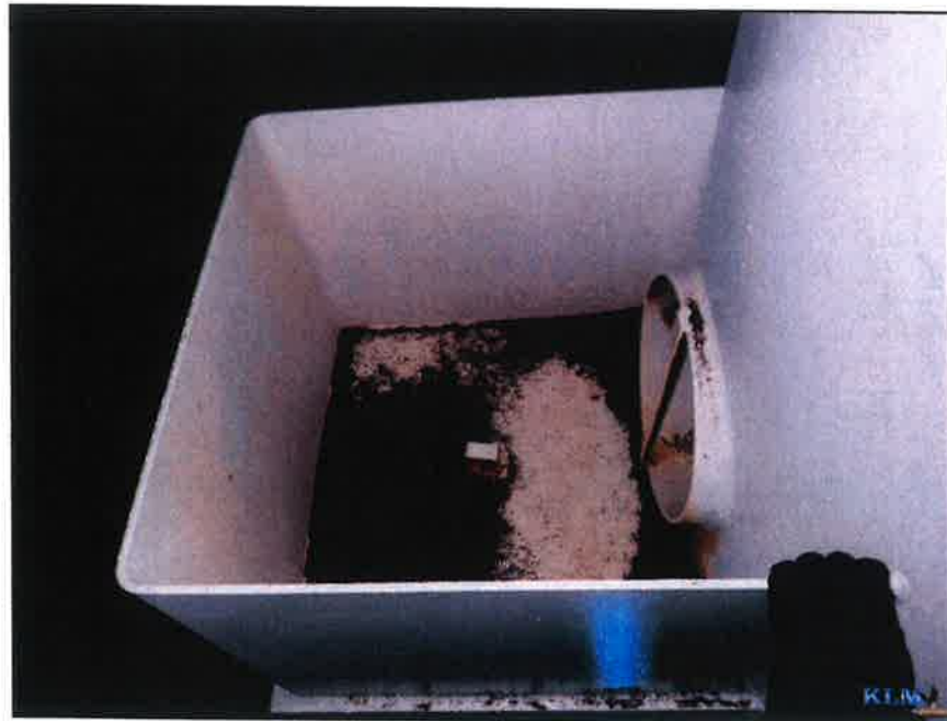
Photo No. 10 Overflow weir box
