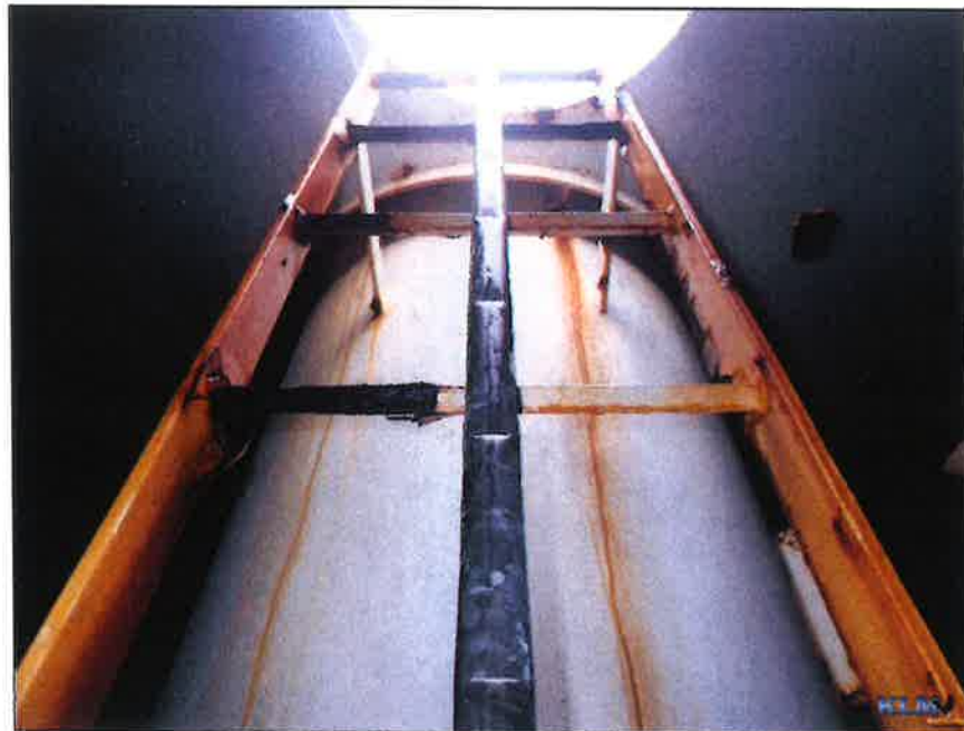
Photo No. 2 Interior wet ladder
