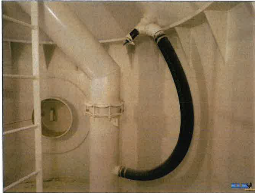
Photo No. 27 Bowl drain valve
