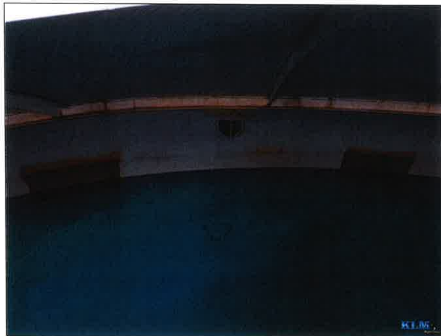
Photo No. 6 Condition of roof and upper shell Overflow pipe inlet visible
