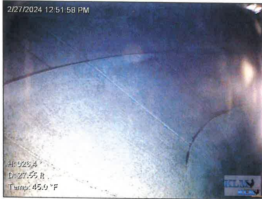
Photo No. 17 Lower torus coating conditions
