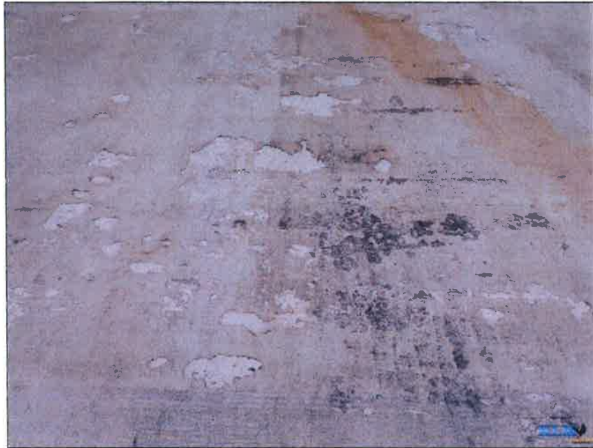
Photo No. 11 Condition of roof coating
