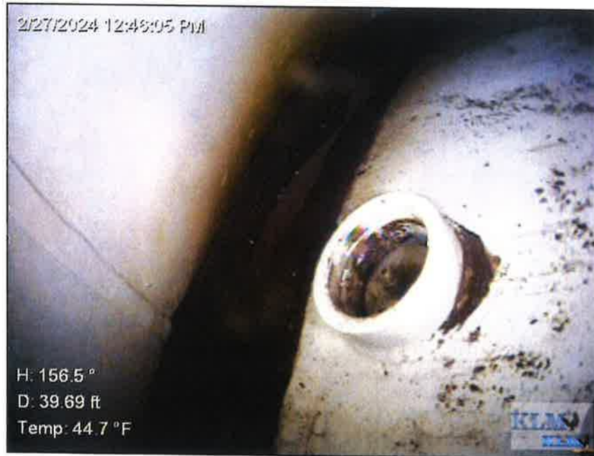
Photo No. 22 Bowl coating conditions Bowl drain coupling visible
