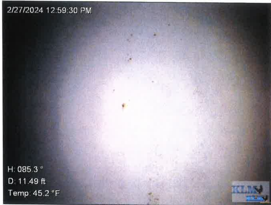
Photo No. 13 Shell coating conditions Pinhole corrosion visible
