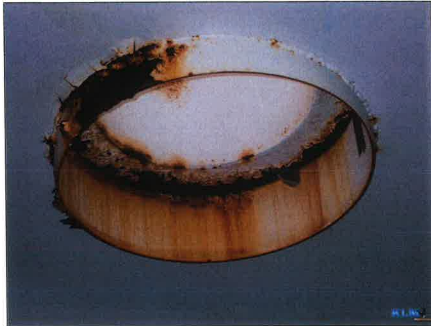
Photo No. 7 Coating failures and corrosion on final vent collar
