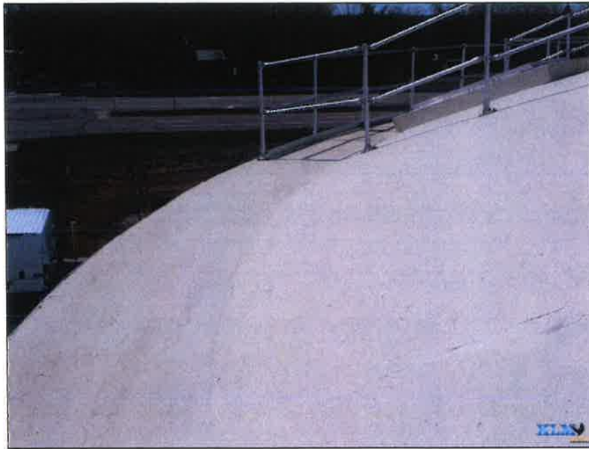
Photo No. 11 Condition of roof coating
