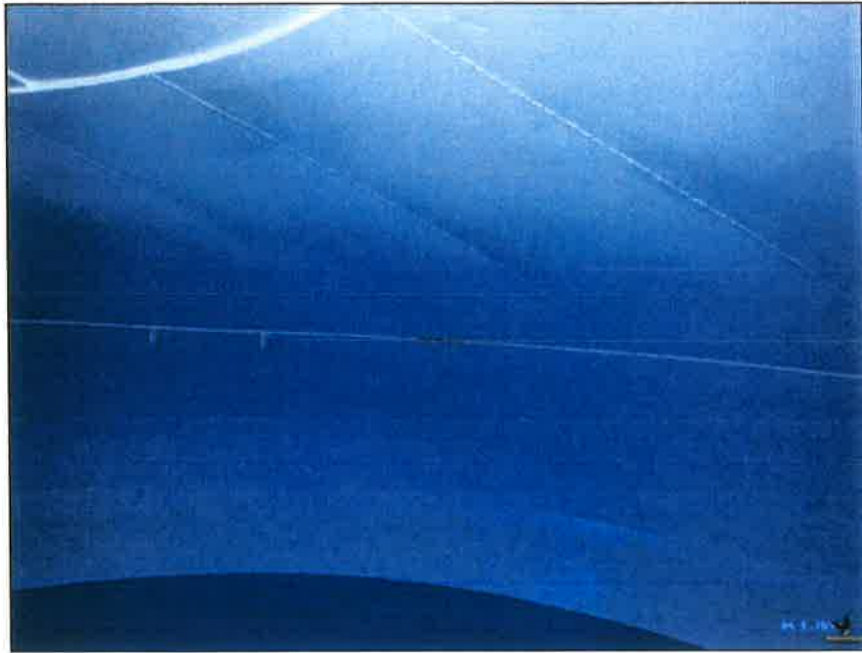
Photo No. 7 Roof and upper torus coating conditions Surface corrosion visible along weld seam
