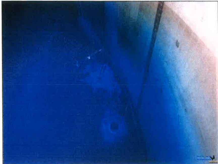
Photo No. 7 View of water compartment Inlet pipe visible
