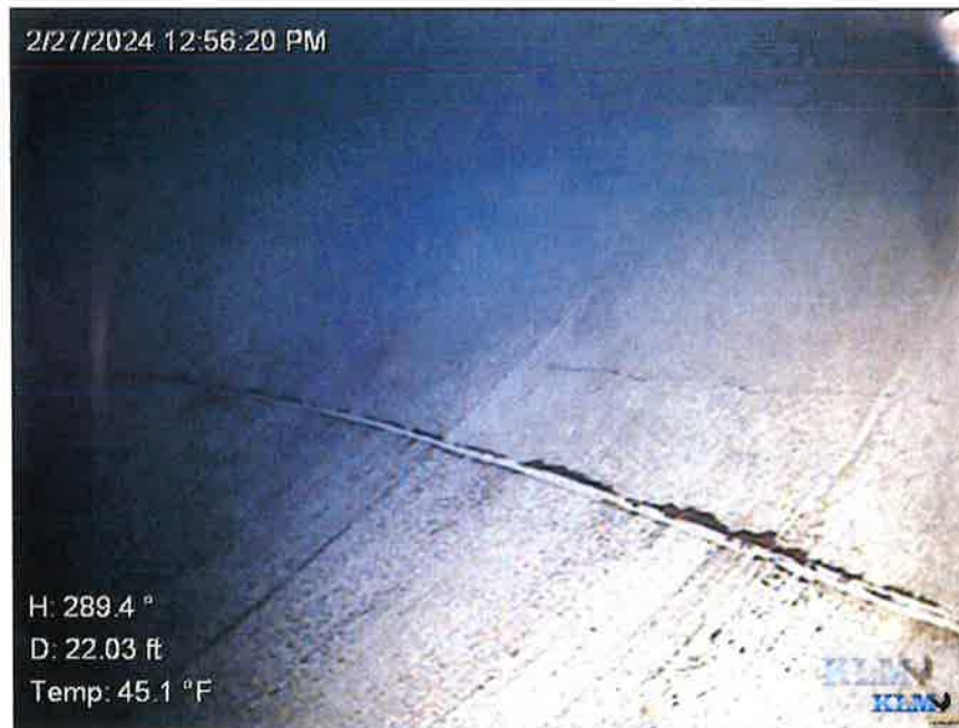
Photo No. 16 Lower torus coating conditions Sediment accumulation visible
