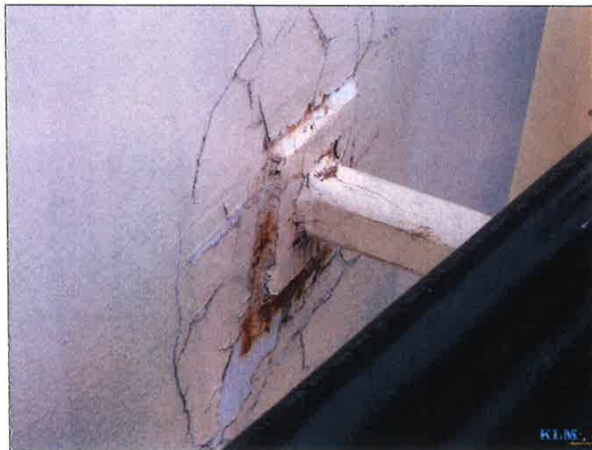
Photo No. 14 Antenna attachment to shell
