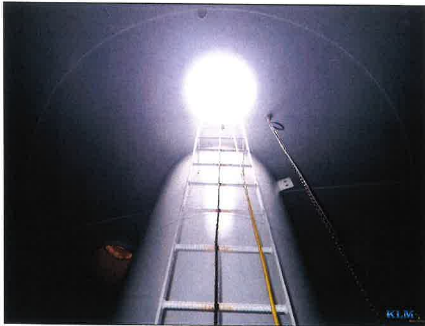
Photo No. 2 View of dollar plate and top of wet access ladder
