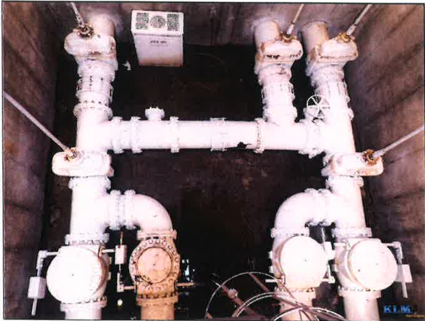
Photo No. 18 View of valve pit
