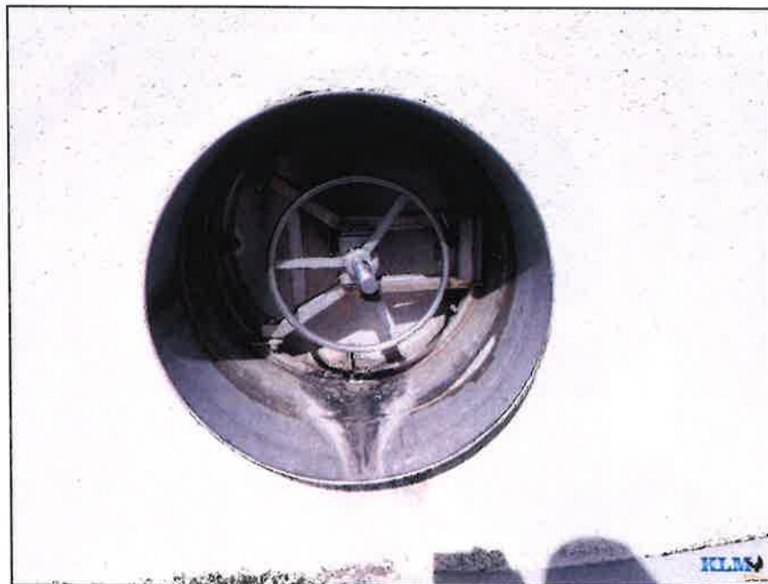
Photo No. 18 Pressure style manway
