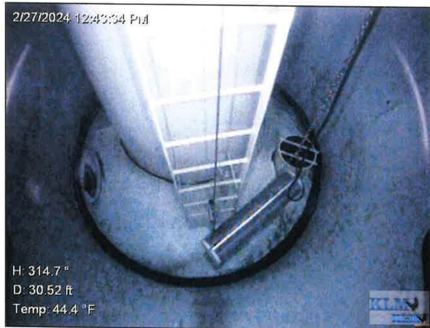
Photo No. 18 Bottom of drywell tube and ladder Submersible mixer visible
