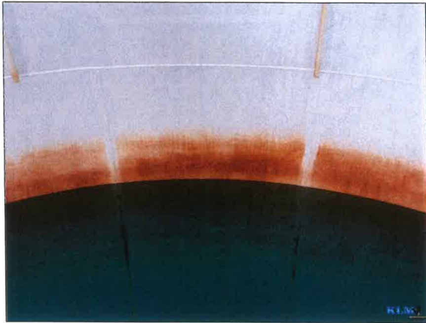
Photo No. 5 Upper torus and shell conditions
