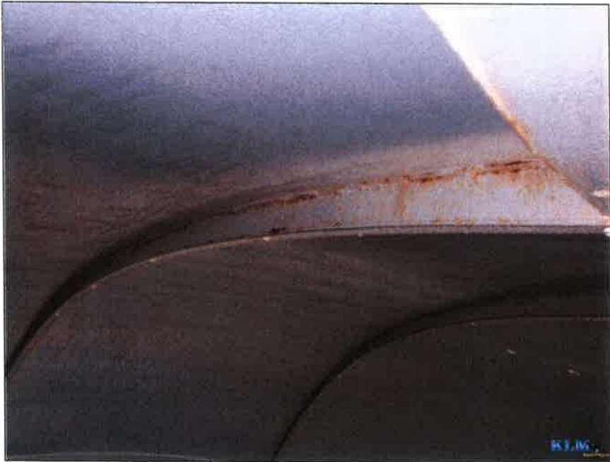
Photo No. 2 Condition of the interior wet roof
