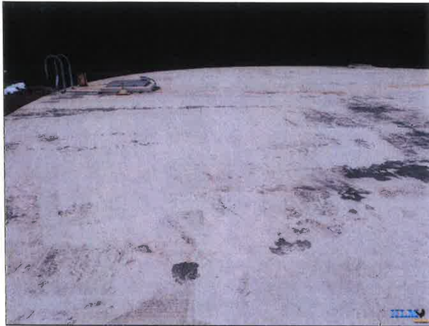
Photo No. 9 Condition of roof coating
