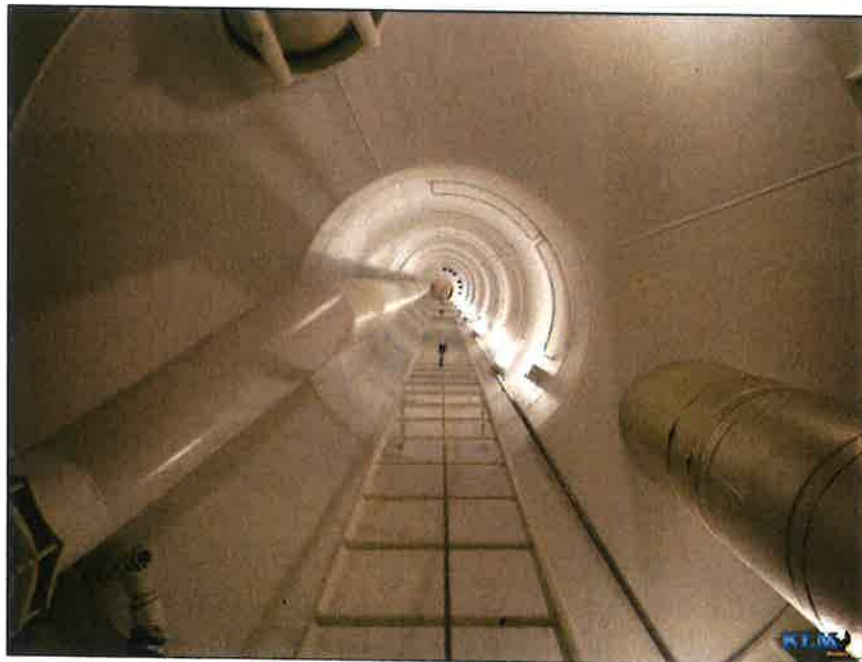
Photo No. 26 Bowl coating conditions
