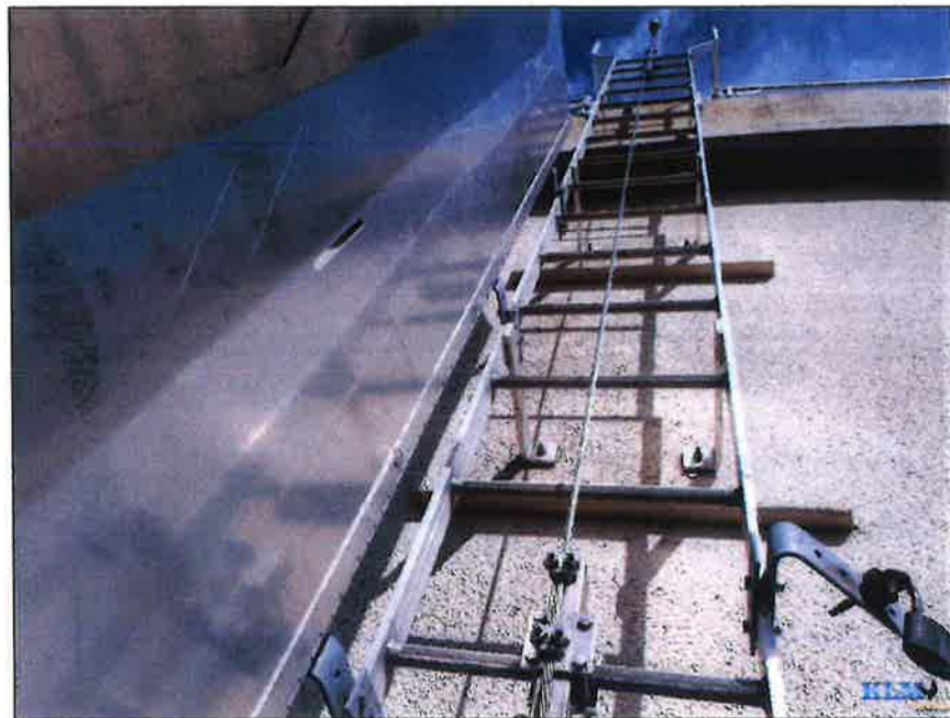
Photo No. 15 Access ladder with anti-climb plate
