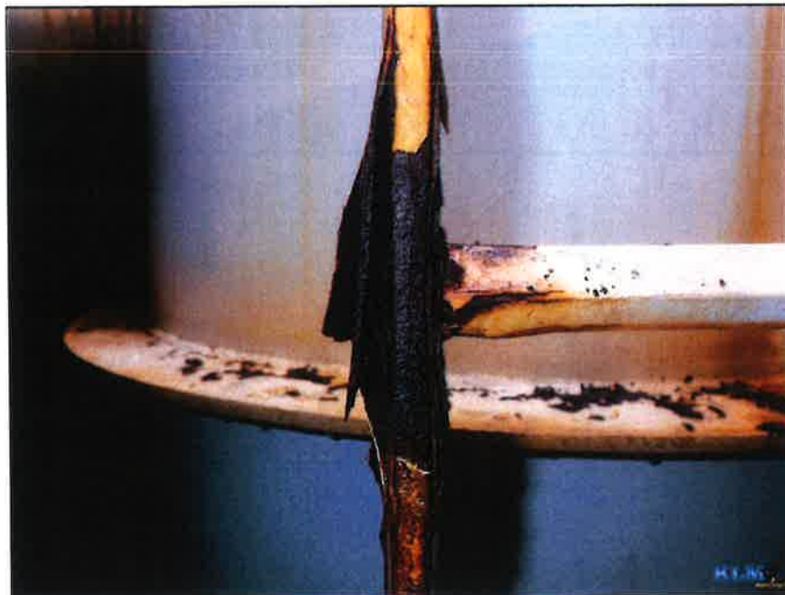
Photo No. 8 Coating failures and corrosion on ladder and drywell tube
