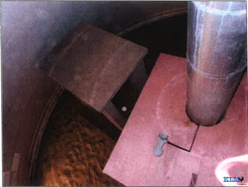
Photo No. 10 Control room and base cone
