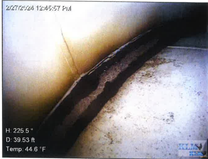
Photo No. 21 Bowl coating conditions
