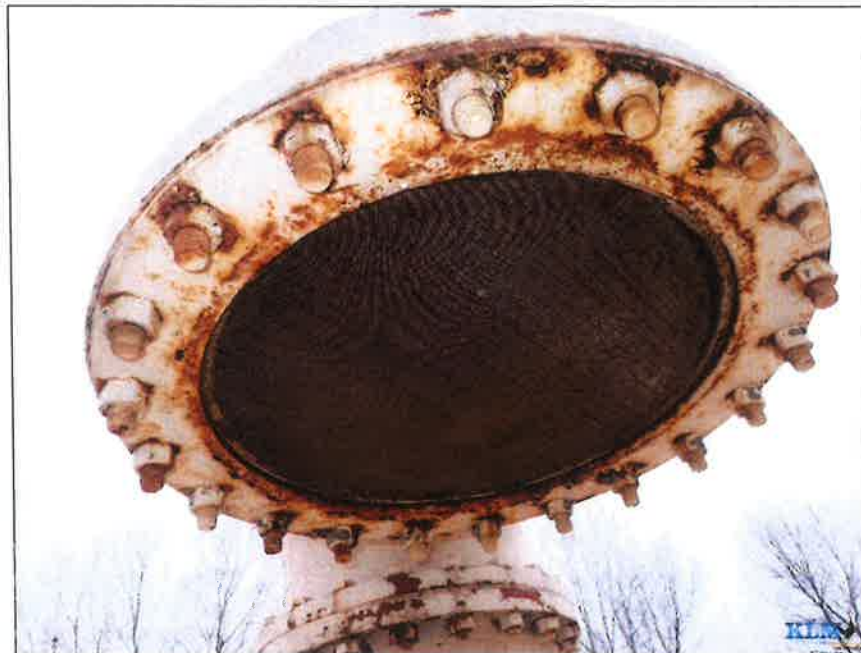
Photo No. 9 Condition of J-vent screen
